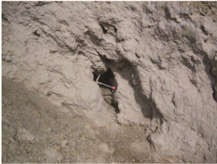
Figure 6: Void in left abutment (note geo-pick for size)
